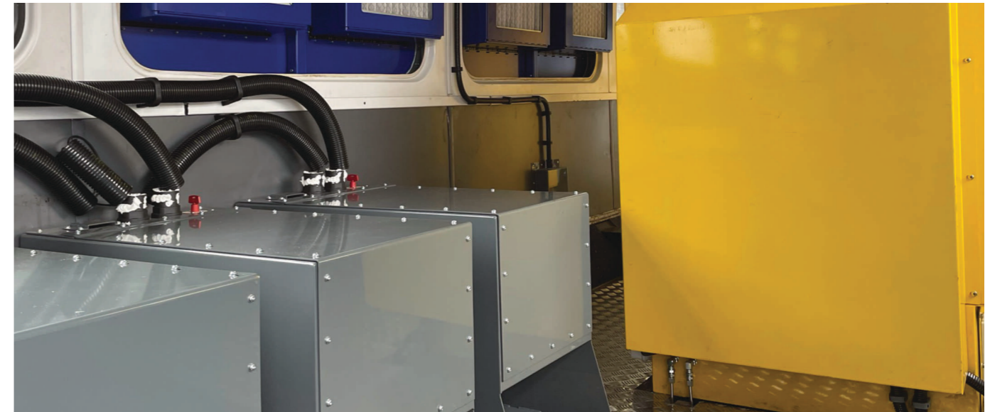
DG8 worked to convert two British Rail Class 153 passenger units into Visual Inspection units for Network Rail
